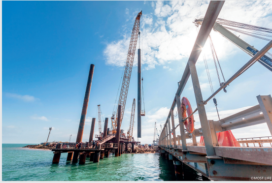
Construction of the worksite for the foundation tube piles immersion, the Kerch Strait, March 2016. Photo from www.most.life
