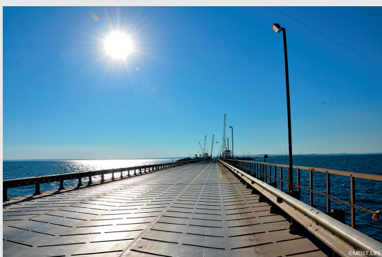
The work bridge from the Tuzla spit to the eponymous island, June 2016. Photo from www.most.life
