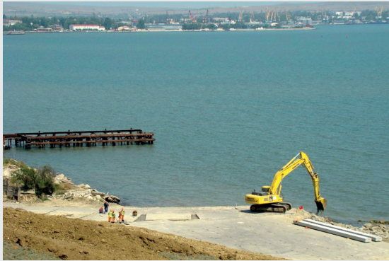
Preparations for the construction of the bridge across the Kerch Strait, August 2015. Photo from kerch-most.ru
