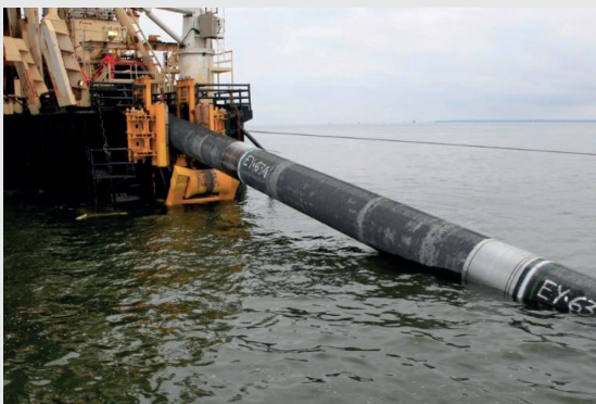
Construction of a gas pipeline from the Krasnodar Territory to Crimea. September 2016. Photo from kerch-most.ru
