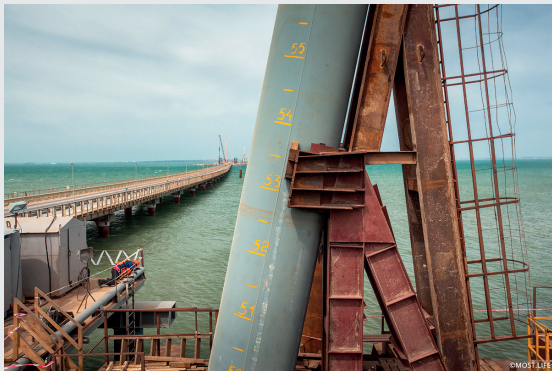
Immersion of the tube under the Kerch Strait car bridge foundation, April 2016. Photo from www.most.life
